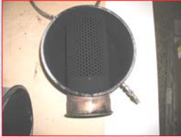
Filter Inlet Section
